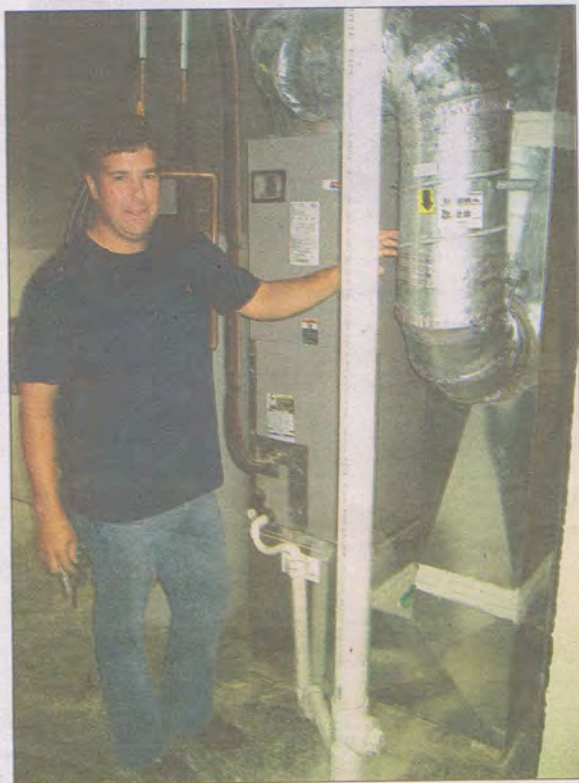
Justin Boyle of Green Valley Builders shows off the HVAC system in one of his Mount Tabor Meadows homes. The conduits are sealed with mastic, rendering them air tight.
